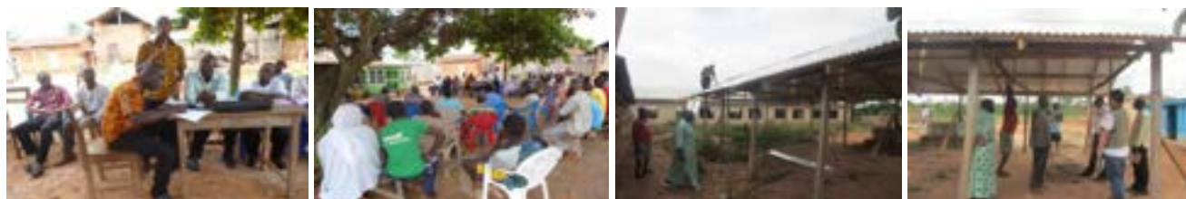
Pasoro PTA General Meeting to raise funds and support for the construction of 2-unit KG classroom. Roofing work been undertaken diligently by a local carpenter under the supervision of SMC/PTA chairpersons and Opinion leader.
